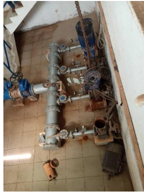
Figure 3 Broken Non-Functioning Essential Water Pumps within Water Treatment Plant, Oti
